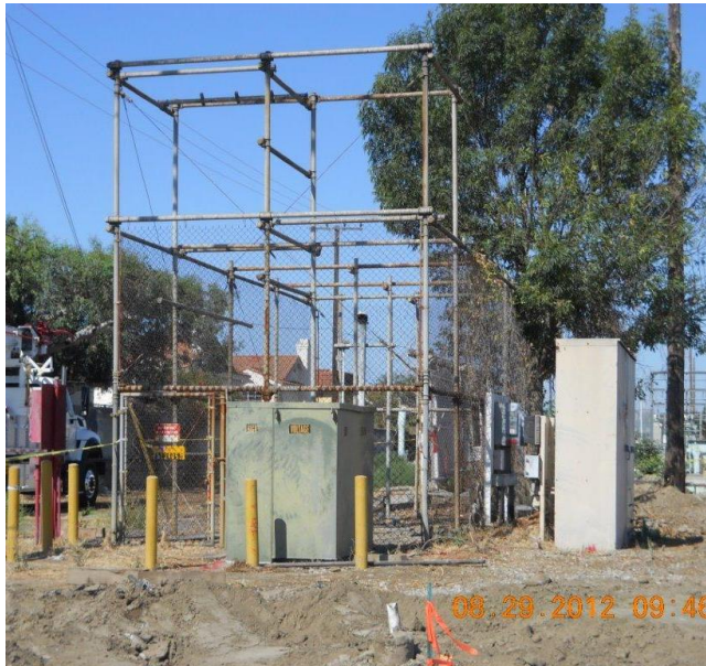
Transformer before demolition
